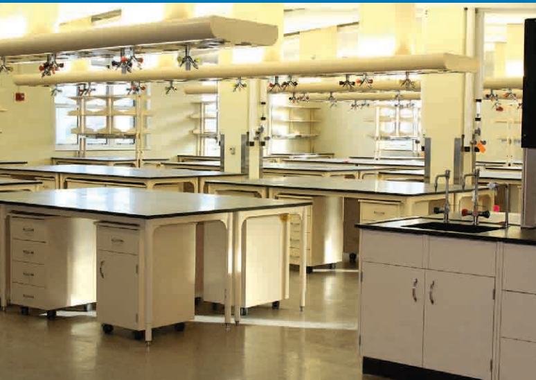
▲ Custom overhead service carriers, mobile cabinets, and fixed steel casework. Project: Carnegie Mellon University, Pittsburg, PA.
