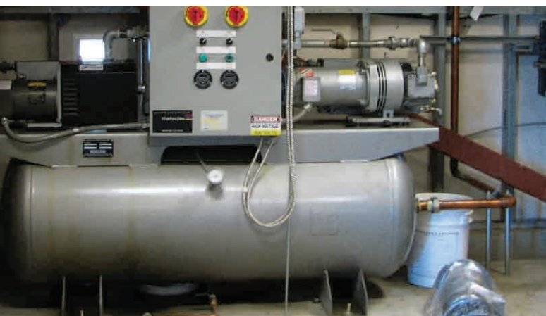
▲ A common configuration for a small central vacuum pumping system: two pumps and a control panel mounted on a ballast tank in the basement.
